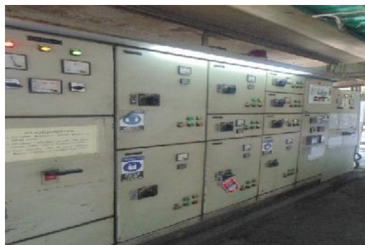
Gambar 2.5 Panel Kontrol Boiler
