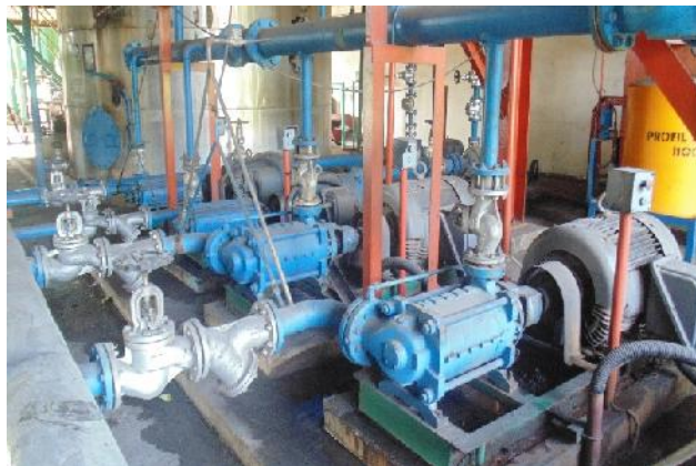
Gambar 2.7 Feed Water Pump
